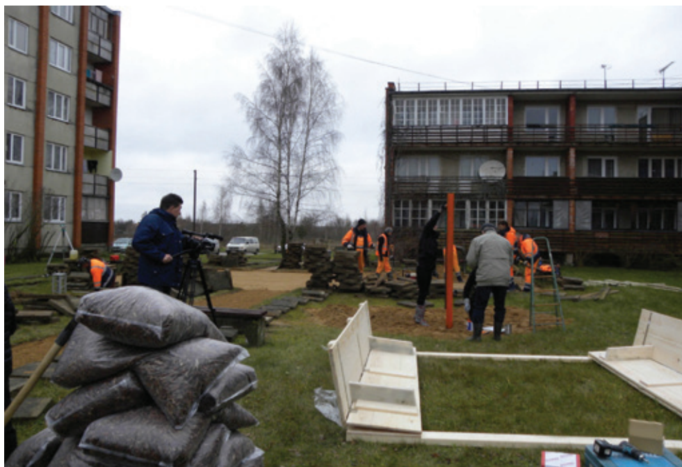
Fig. 14. Improvement works in 2, 2a, 4 Nameja Street. [Source: photo from Una Īle's private archive, 2013]
