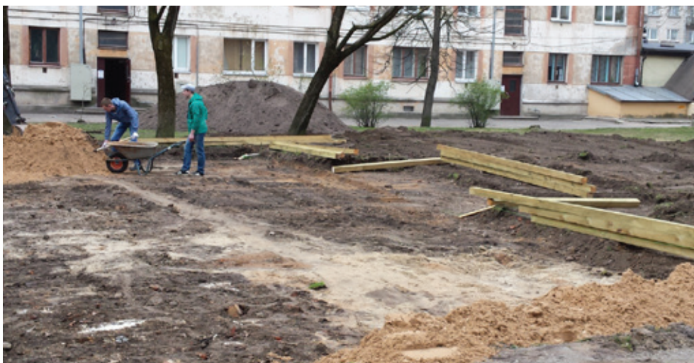
Fig. 12. Installation works in the future playground area. [Source: photo from Una Īle's private archive, 2015]
